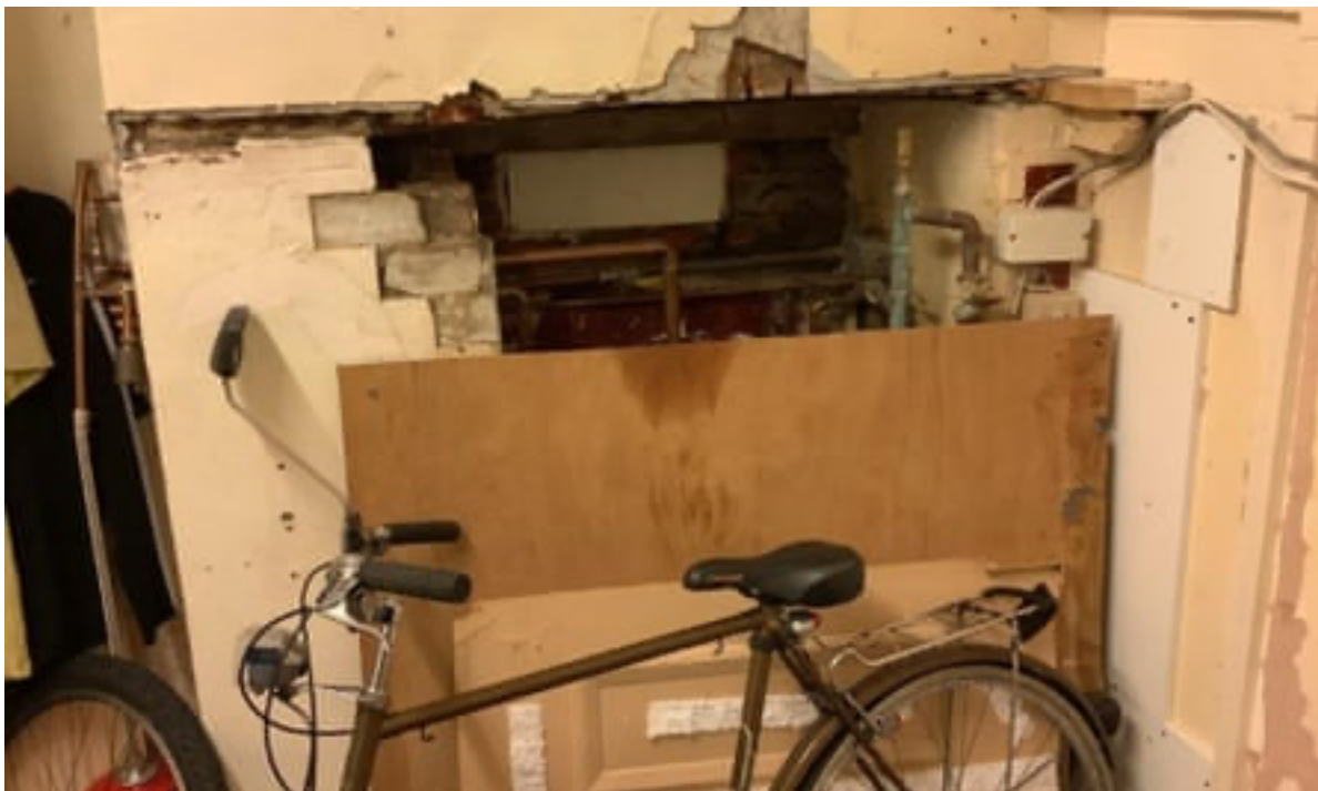
A damaged chimney breast in a HMO in Southend. Photograph: Southend-on-Sea council
